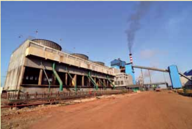
Co-gen cooling Tower
